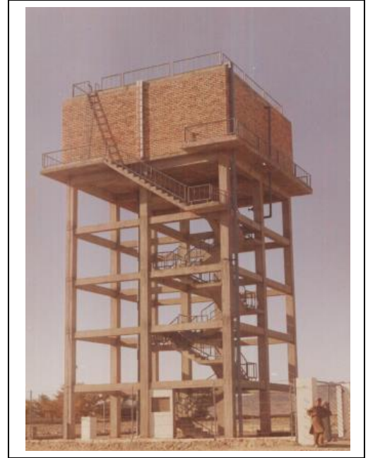
Over Head Water Reservoir 50000 Gln Capacity
