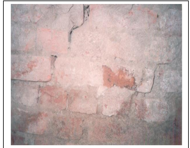
Cracks developed in the Wall
